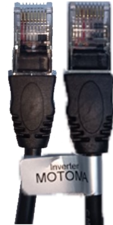
BMS Communication Cable
